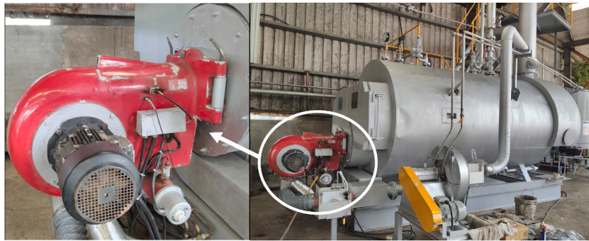
Fig. 3. Picture of Experimental boiler and apparatus.
